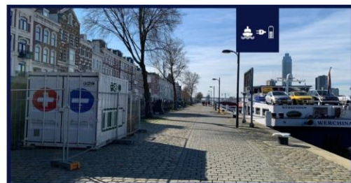
Shore battery for inland vessels
